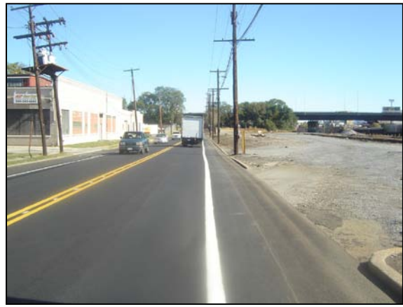
Bicycle lane on Shenandoah Avenue installed as part of the 2011 annual paving program
