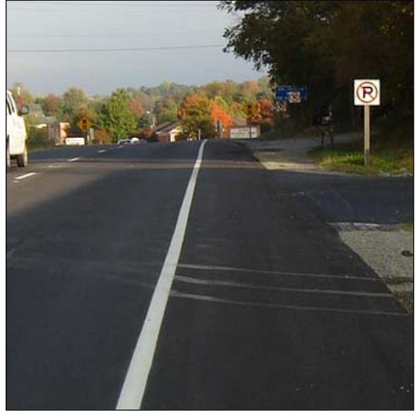
Paved shoulder on US 220 North in the Daleville area of Botetourt County
